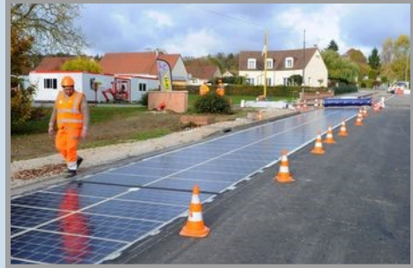
Wattway's solar road in Tourouvre
